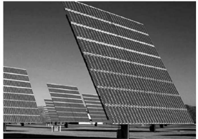
Typical Solar PV Panel Installation
