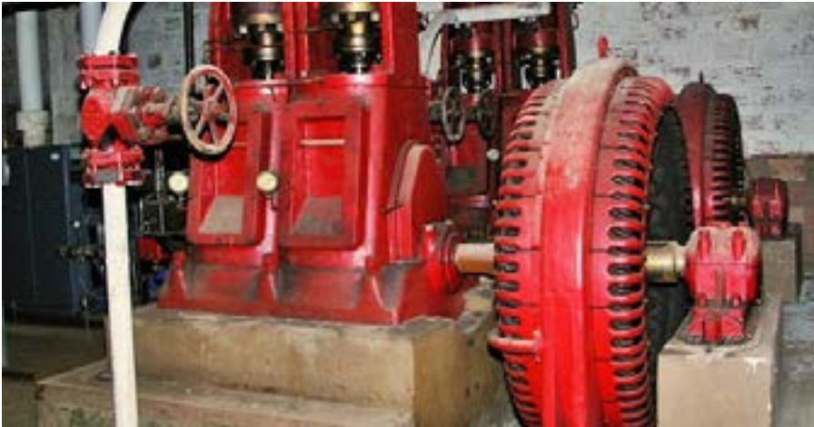
Fig 1: A pair of ancient Carbon Dioxide air conditioning compressors, powered by two antique 150 horsepower open frame synchronous motors. This type of A/C system dates to the 1930's.
